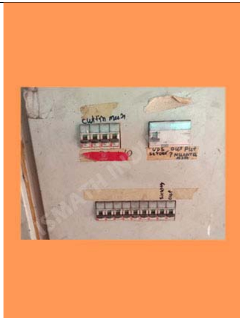
Lighting Distributions Board
